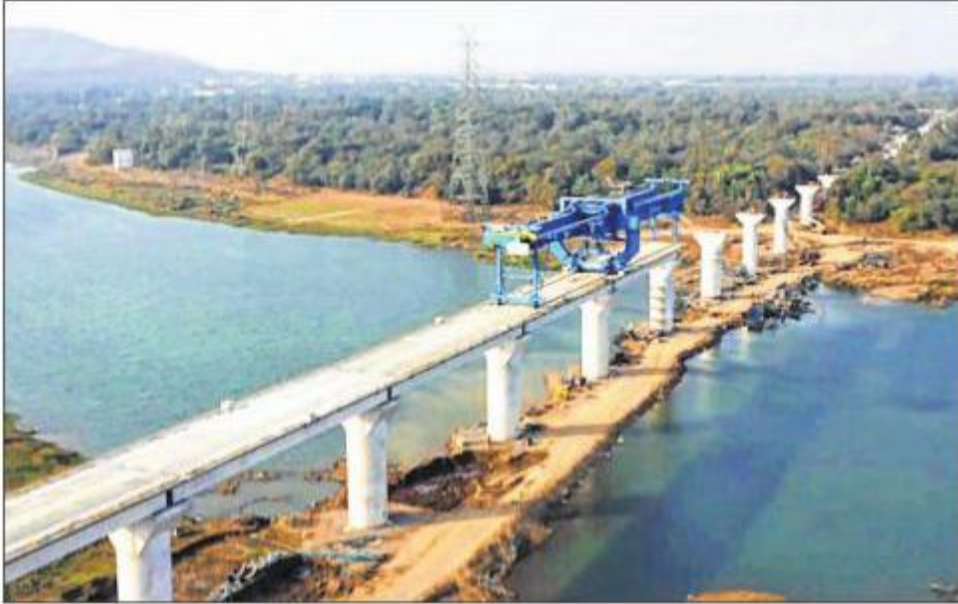
Construction of the first river bridge of the Mumbai-Ahmedabad High Speed Rail Corridor over Par River in Valsad is in full swing.
